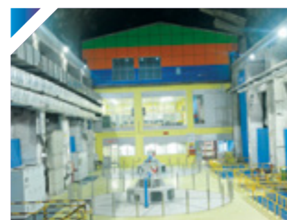
Now: T.G HALL with CFL & LED lighting at Dikchu HEP
