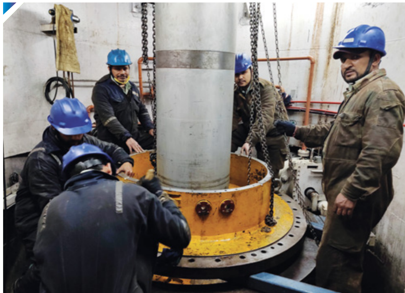
We always adopt, Reduce, Reuse, Recycle, Repair, Refuse during O&M of our assets.
